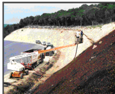
Application of a 2 inch-thick compost blanket to a 1:1 rock slope using a pneumatic blower (Austin, Texas, 2002). Source: McCoy, Texas Commission on Environmental Quality (TECQ), 2005
