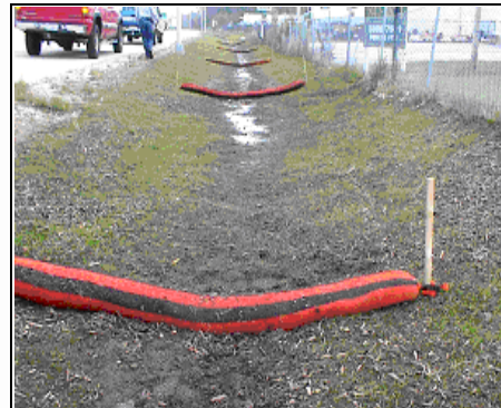
Installation of filter socks in a road ditch by Earth Corps for Indiana Department of Transportation. The filter socks will be staked through the center. Source: Filtrexx International, LLC.
