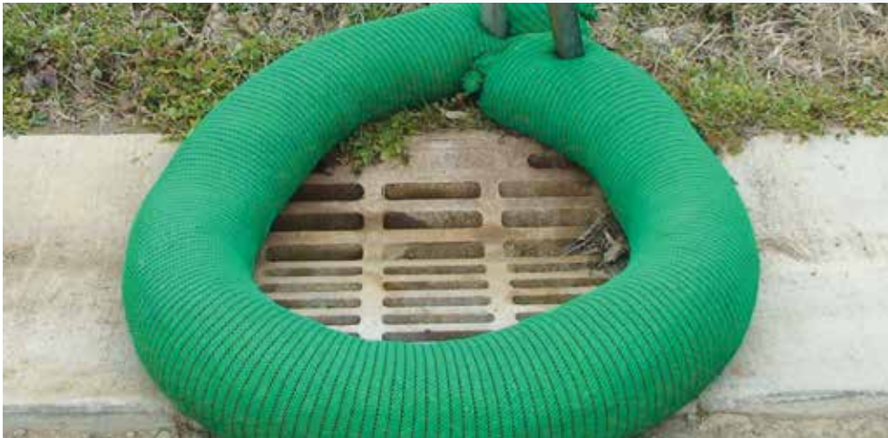
Filters runoff water as it passes through by allowing water to temporarily pond
