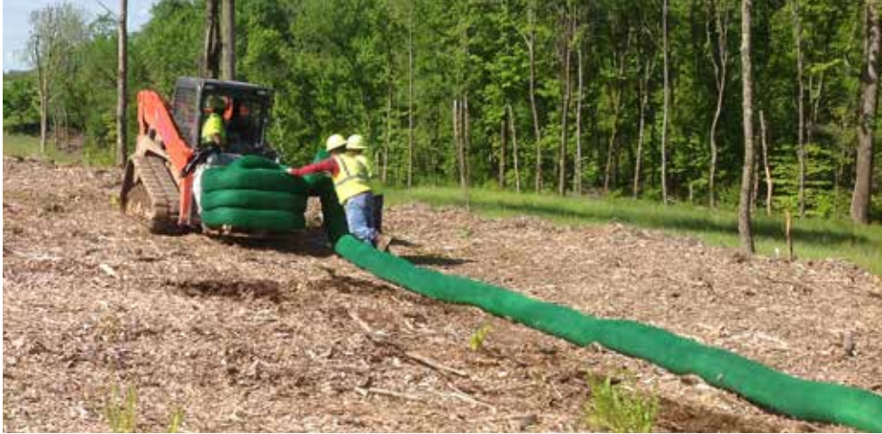
The best BMP available—Filtrexx® SiltSoxx™ let water flow through while keeping sediment behind the Soxx™
