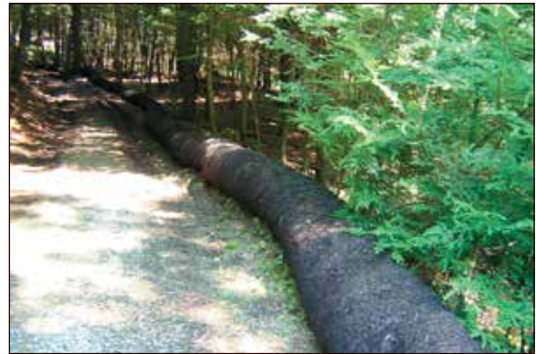
24 in Runoff Diversion for High Storm Flow
