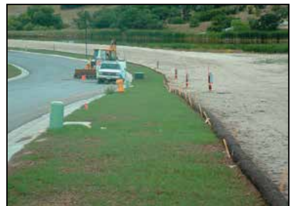
Filter Strip with a SiltSoxx™
