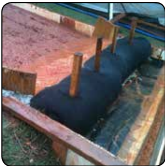
Fig. 2: 12" SiltSoxx™ (97% Removal Efficiency)
