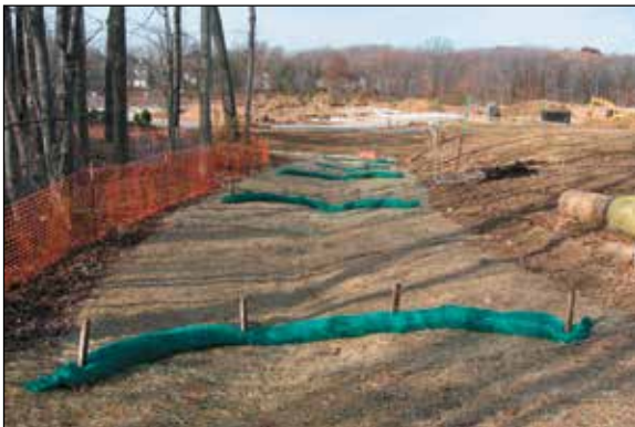
Use as Speed Bumps to Slow Storm Water Velocity
