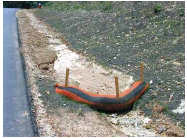
Figure 3 Compost filter sock check dam
