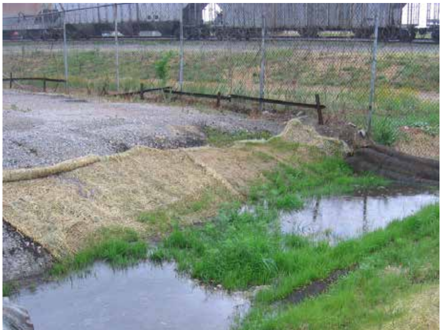
Figure 2. Filtrex ® Filtration system was installed April 20th, 2007, to evaluate their performance on chemical oxygen demand (COD), total suspended solids (TSS), and oil and grease in the storm water effluent from CWS Outfall #2.
